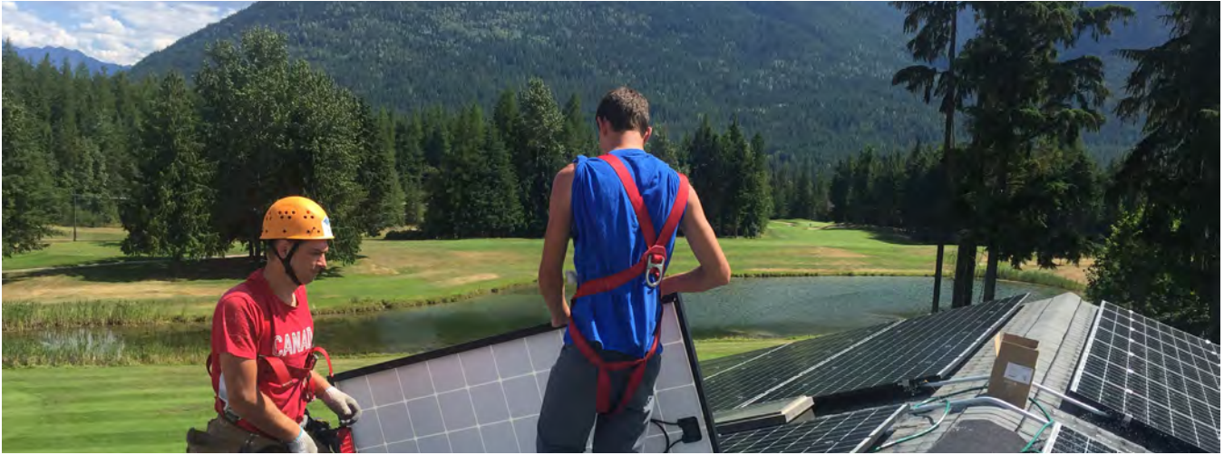
Solar PV installation at Balfour Golf Course clubhouse, B.C. Photo: Dave Lovekin
