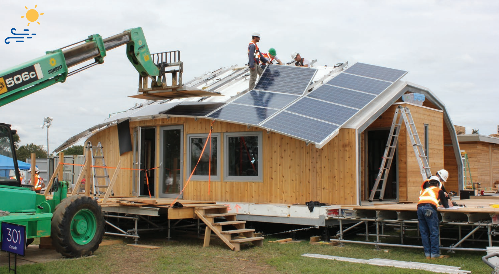
Installing solar panels on the roof of a Traditional Living house at the University of Calgary. Photo: Carol Anna/U.S. Department of Energy
